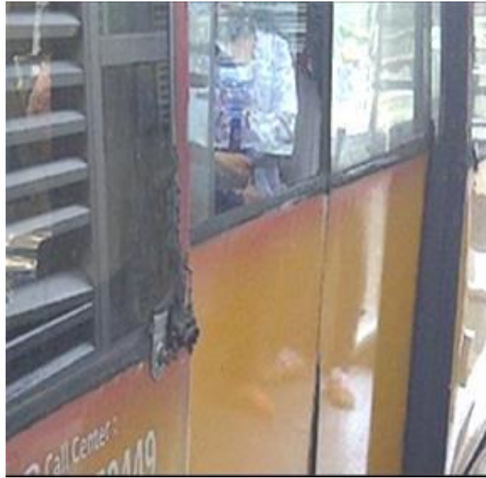
Figure 1: Crack on column structure at the window corner of Busway
