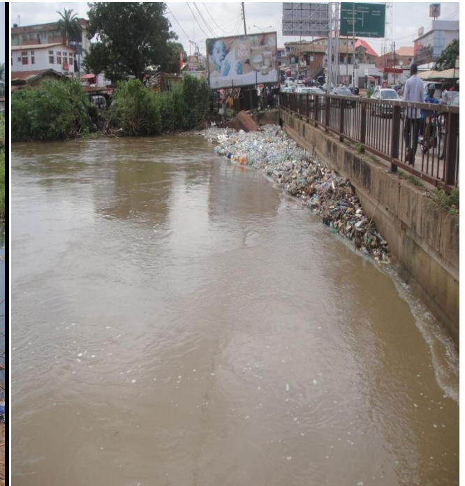
Figure 4b: River channel capacity reduced at Unity road due to sedimentation and vegetation (after rainfall).
