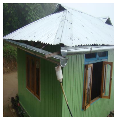
Fig.7: Roof top water harvesting at Lava (2000 m asl)
